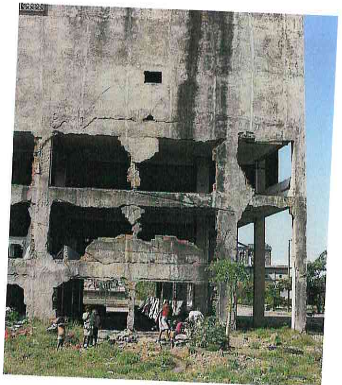
Earthquake damage, Managua
