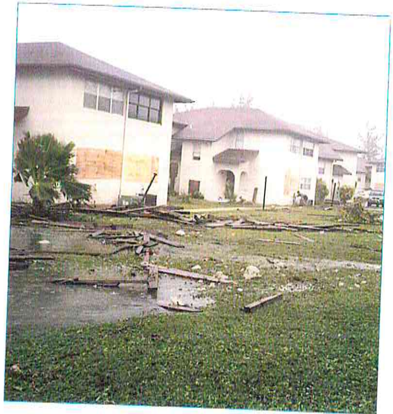
Damage caused by Hurricane Mitch, 1998
